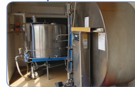
Milk room with parts of the cooling tank and buffer tank.
